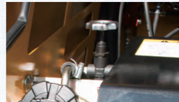
▲ Emergency vessel reset valve
